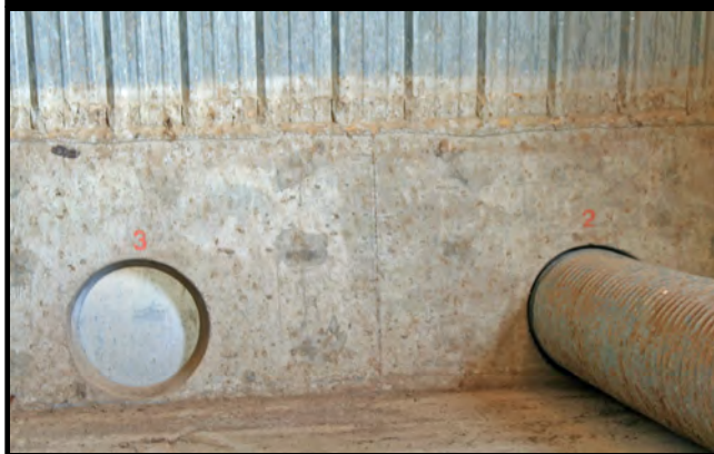
Figure 2.6. Ventilation duct openings from plenum chamber.
