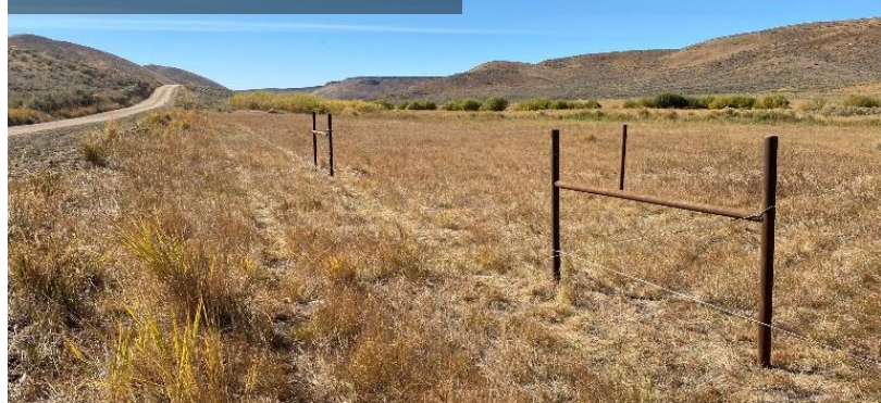
METAL H-BRACE READY FOR WIRE
